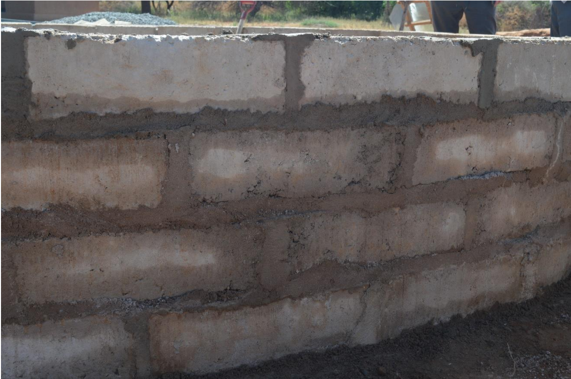
Figure 62: Wall progress made from previous Thursday. Top block done in the morning
