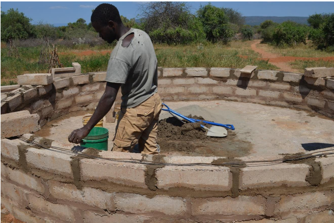
Figure 65: Laying wire and holding it down with blocks. Mixing mortar on slab of tank
