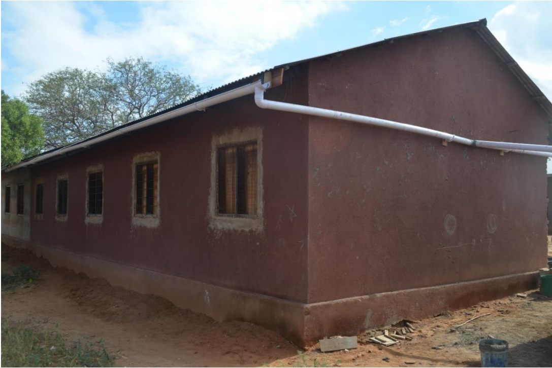
Figure 74: Gutters and Piping Connections
