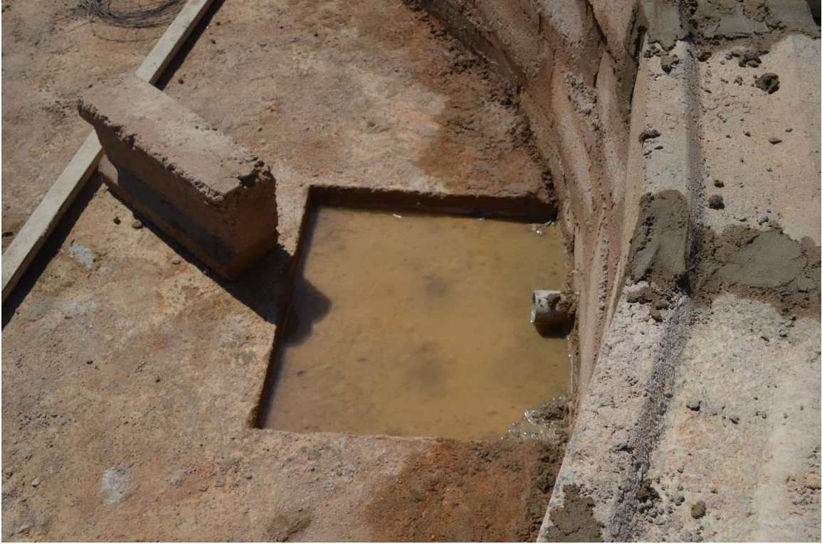
Figure 68: Clean out installment on inside of tank
