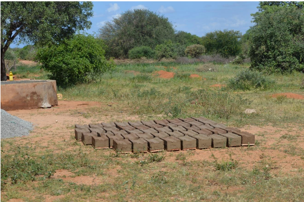
Figure 44: Laying out bricks to cure. 65 were made the first day, over 100 were made the next block making days
