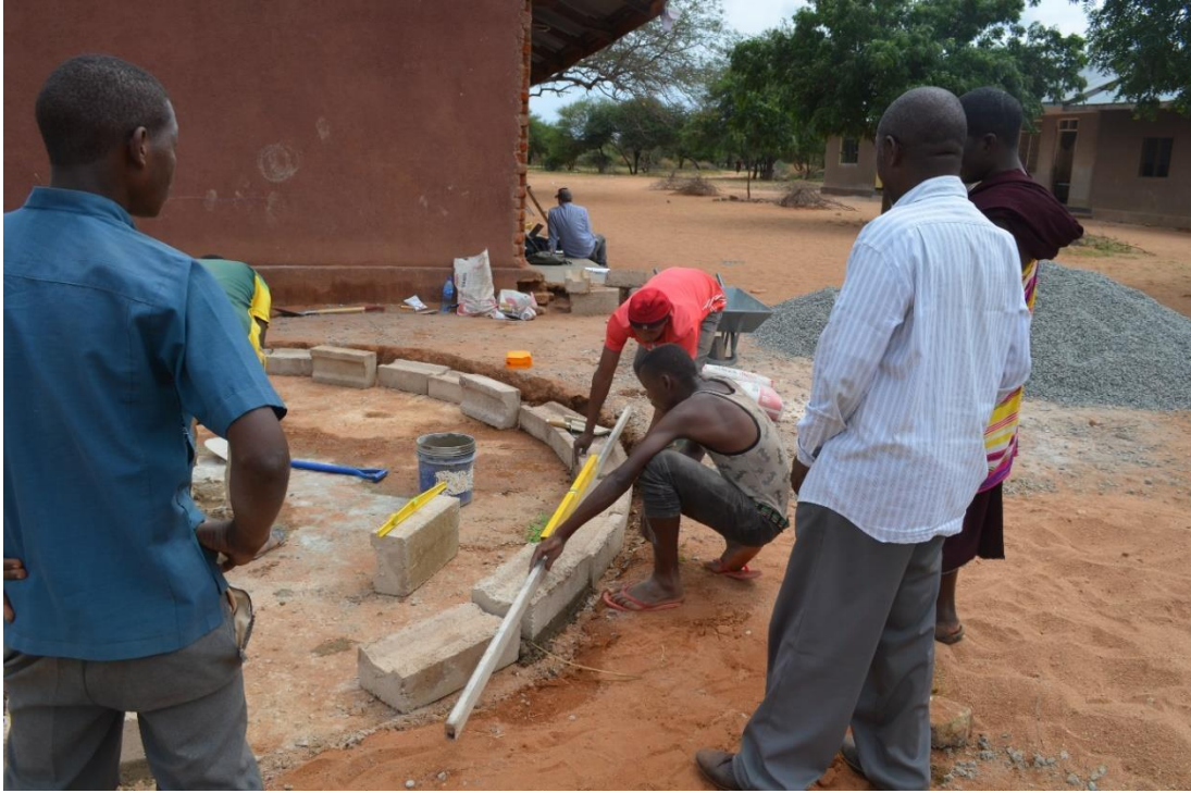
Figure 59: Began setting first course on mortar. Levelled every third block and then came back for the blocks in between.
