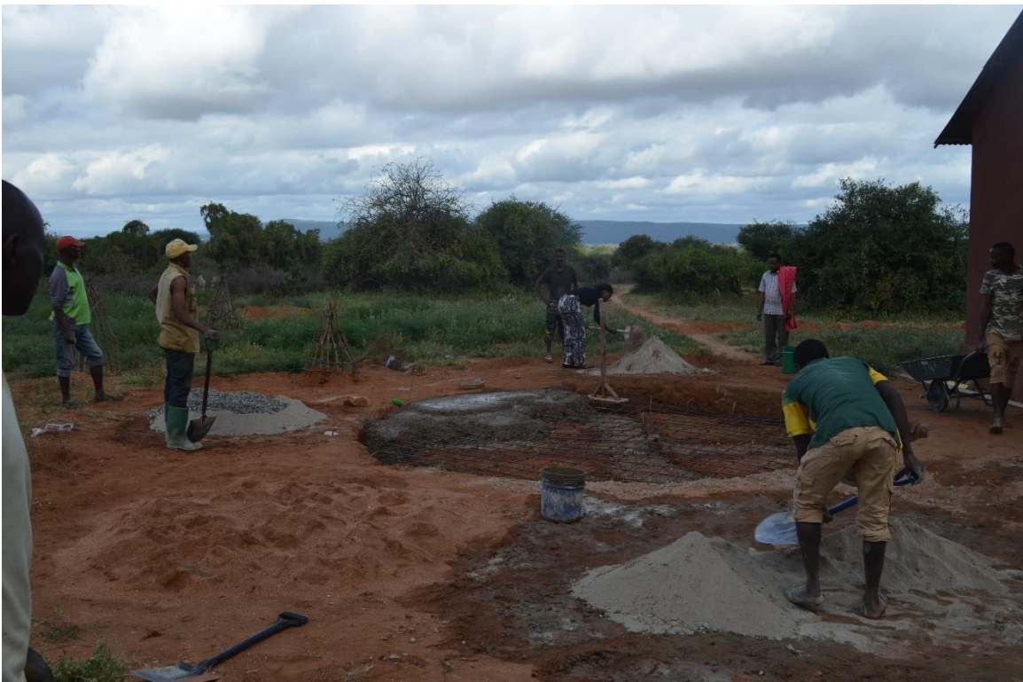
Figure 48: Decided to split batch up into thirds at different locations around the foundation.
