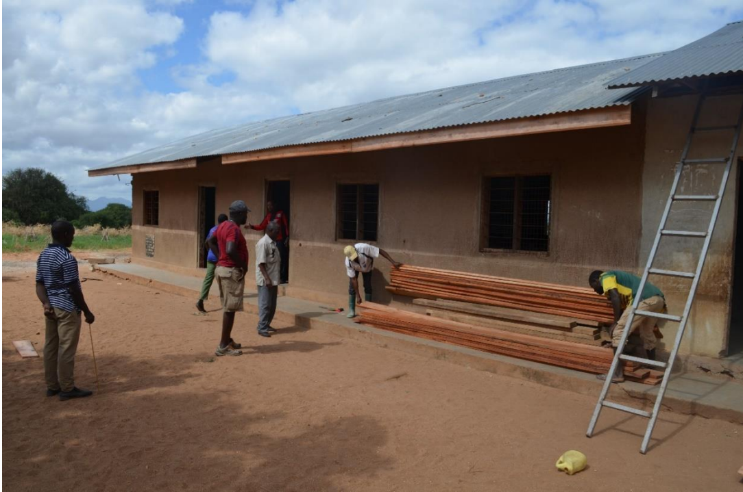
Figure 52: Facia installed upon arrival, was short on sanded facia board
