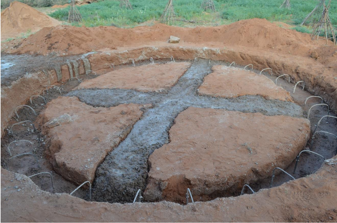
Figure 40: Completed first pour. Beams were filled higher with leftover concrete and stirrups were left out for cold joint.
