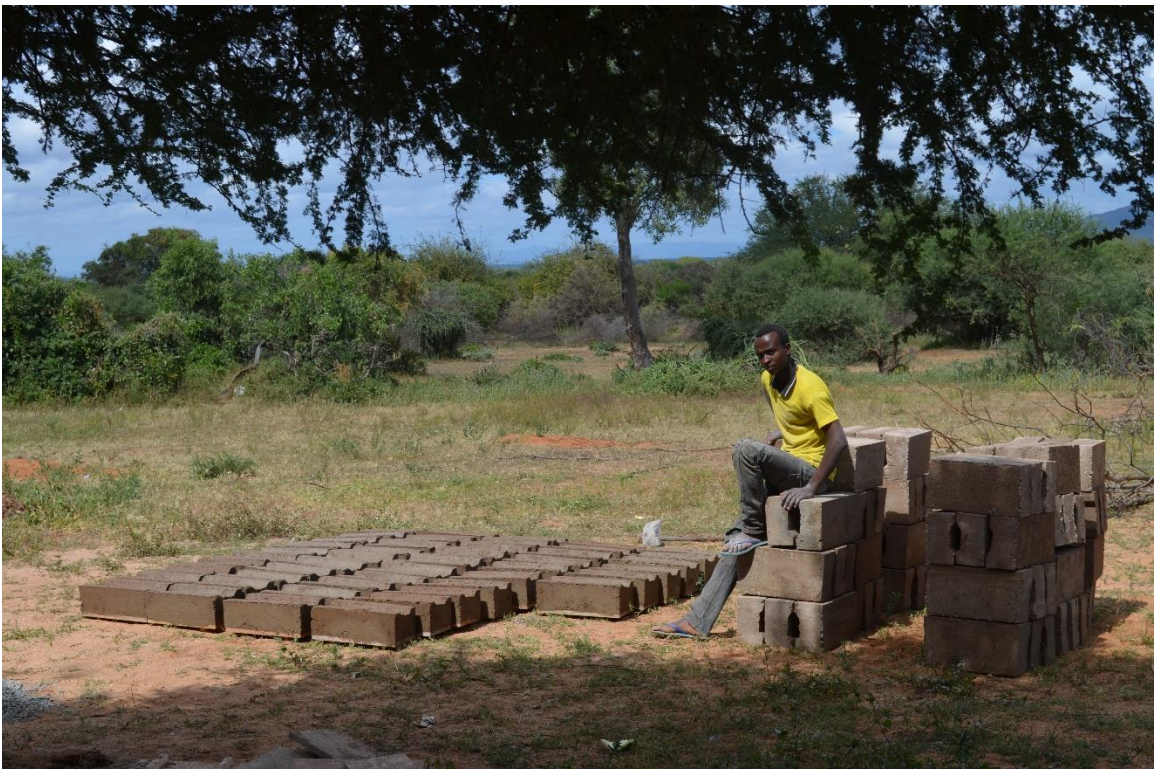
Figure 55: Continuing of block making while the fascia board was installed and were short on fascia board
