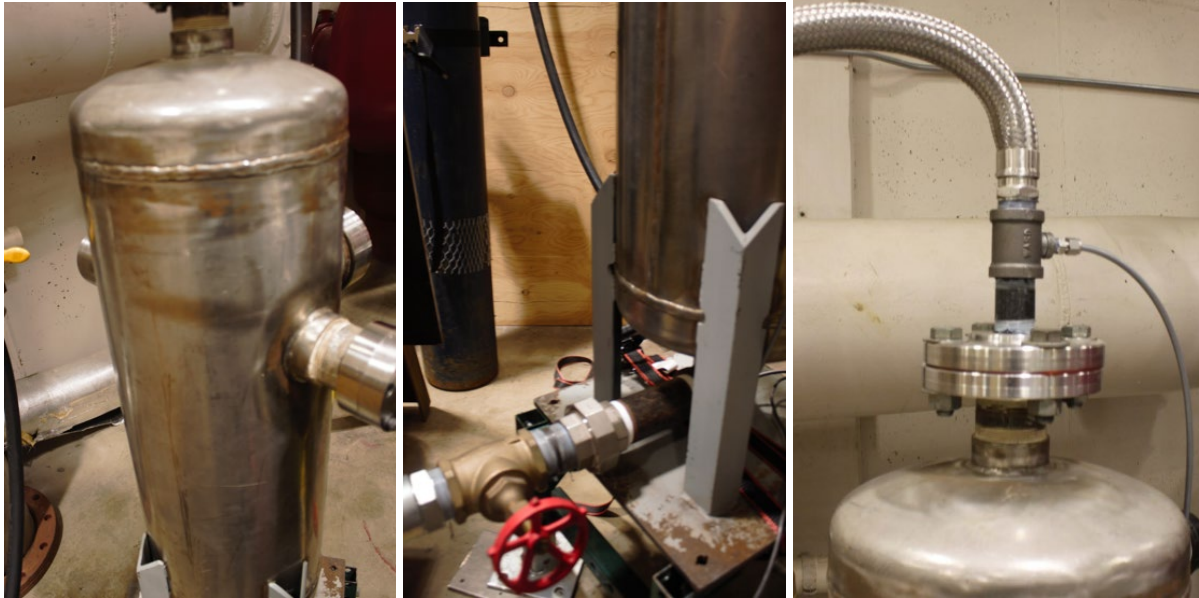
Figure 30: Exhaust Containment Tank with the Dilution Air Line shown in the middle and the stainless-steel line to the vacuum injector on the left
