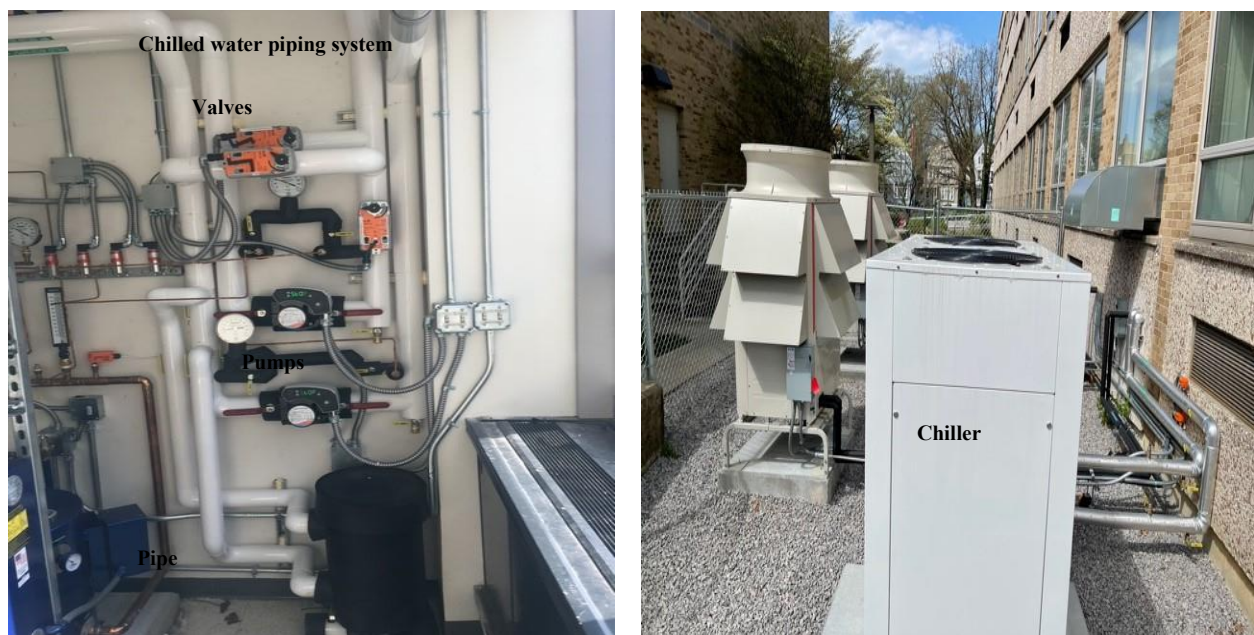
Figure 27. Chilled water central plant pictures.
