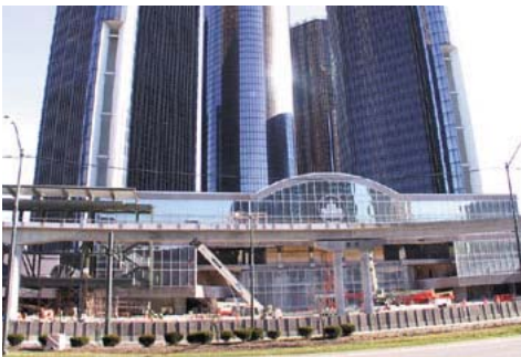
Figure 3.36 Renaissance Center – Detroit, Michigan – street level experience (currently under renovation in photograph) – concrete berms being replaced by full height glazing
