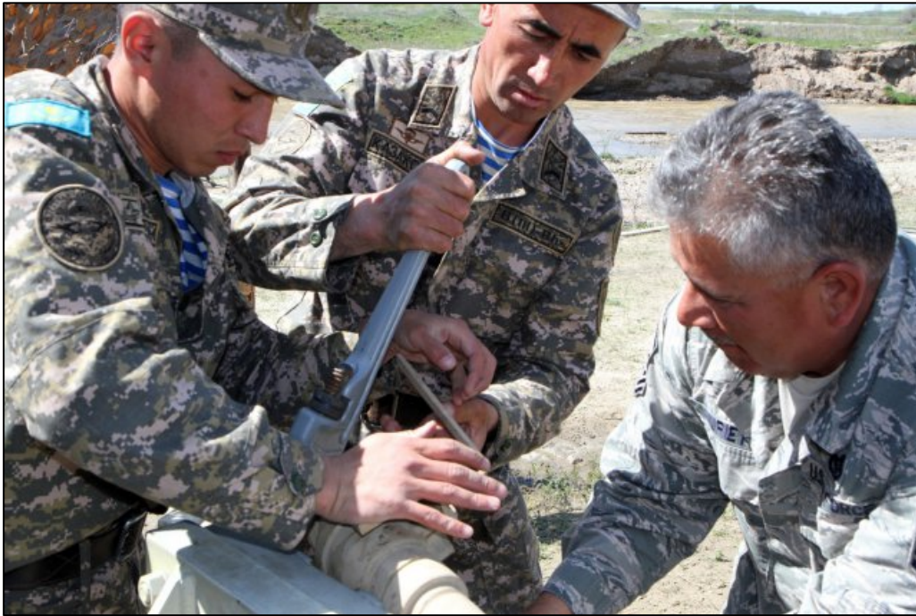
Figure 7. Air Force Msgt Alberto Murietta, civil engineer operations noncommissioned officer with 161st Civil Engineer Squadron, helps two soldiers from the Kazakhstan Peacekeeping Battalion fix a pipe on their Reverse Osmosis Water Purification Unit at Illisky Training Center during preparation for Steppe Eagle 16. Steppe Eagle is one of many opportunities members of the Arizona National Guard use to grow their relationship with Kazakhstan as part of the State Partnership Program. (U.S. Army photo by Maj. Chris Brautigam, USARCENT Public Affairs) (Photo Credit: Maj. Christopher Brautigam)
