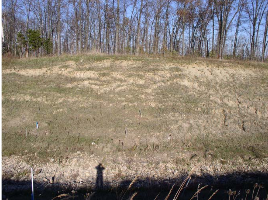
Figure 4.7: Scarps and erosion on the northeast slope, November 2005.
