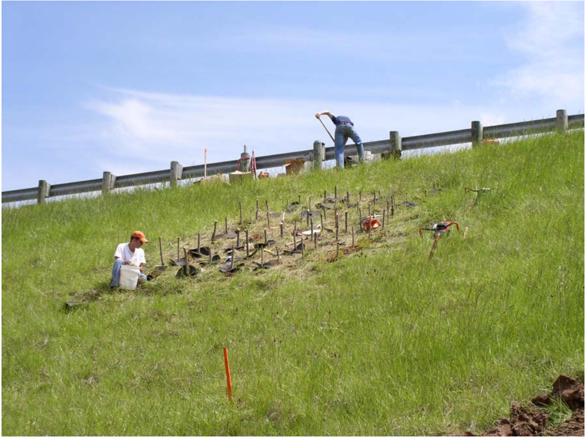
Figure 5.31: Muskingum County upper live pole plot during installation near STA 1+00 (June 2005). (see Figure 5.7 for STA reference)
