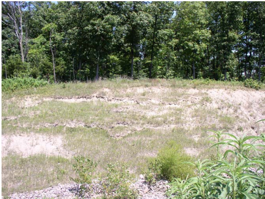
Figure 4.4: Scarps and erosion on the northeast slope, August 2004.
