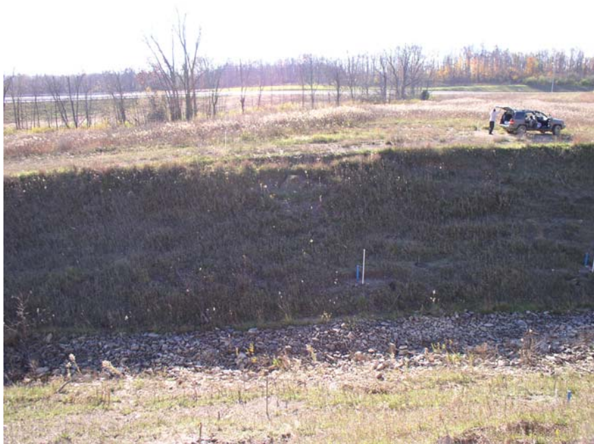
Figure 4.8: Scarps and erosion on the southwest slope, November 2005.
