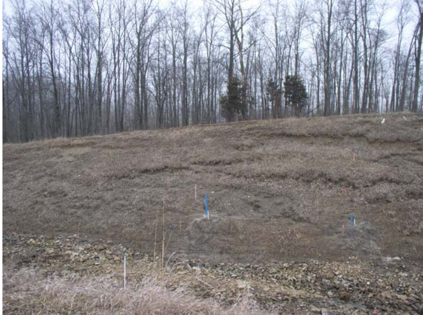
Figure 4.5: Scarps and erosion on the northeast slope, February 2005.
