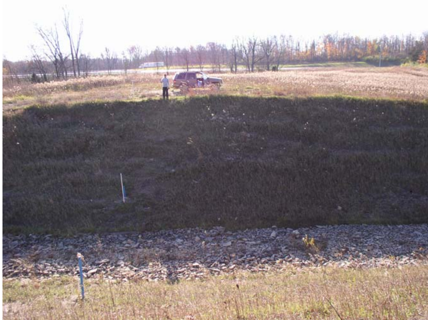
Figure 4.9: Scarps and erosion on the southwest slope, November 2005.
