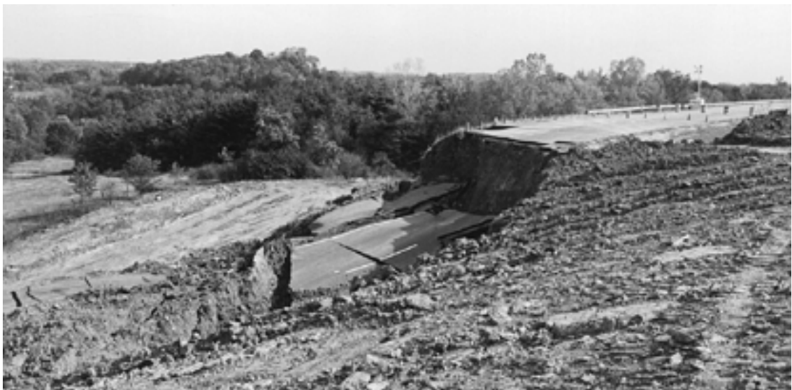
Figure 5.6: Landslide in Conemaugh formation in 1986 destroyed the westbound lanes of I-70 near New Concord, Guernsey County. (Photo from DeLong (1996))
