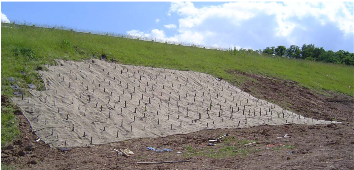
Figure 5.28: Muskingum County main live pole plot after installation near STA 0+75 (June 2005). (see Figure 5.7 for STA reference)
