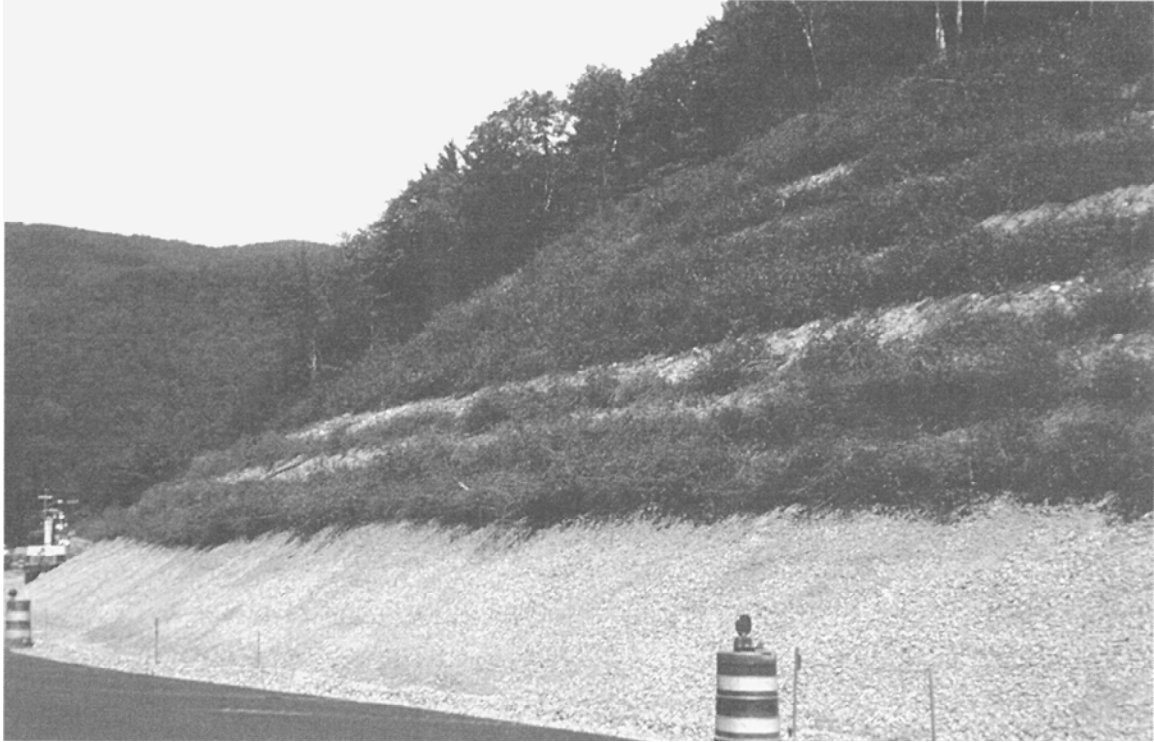
Figure 2.7: Brushlayer fill during first growing season – Greenfield road near the village of Colrain in Massachusetts. Brushlayers have rooted and leafed out. (Gray and Sotir 1996)
