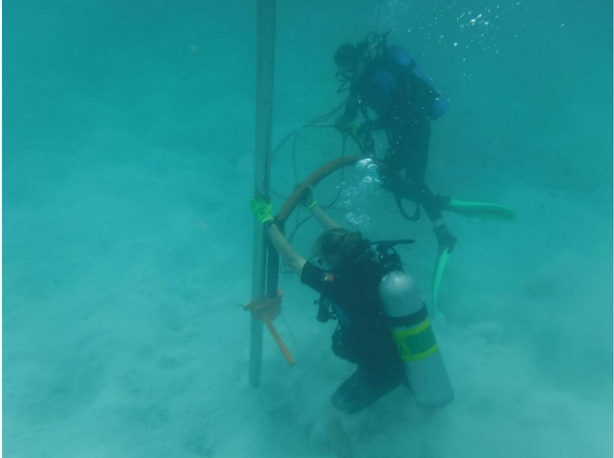
Figure 9: Karla Parsons Hubbard (lower) and Rebekah Shepard (higher) hold the core pipe steady before switching on the concrete vibrator. Photo taken by Rowan Lee during field research in Great Pond Bay, USVI 2018.
