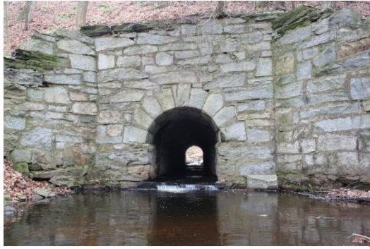
Figure 21 Example of culvert type fish passage. Notice how it chokes down the actual stream width. It becomes a physical barrier during low flow periods. (photo from. www.obsidianportal.com )
