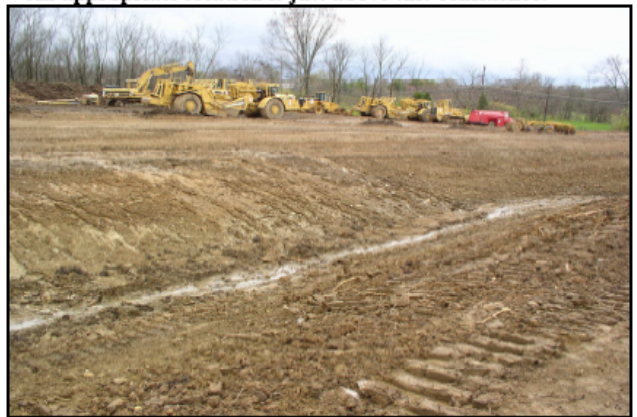
Figure 4. Existing drainage route exposed and erosion rills forming on slopes.
