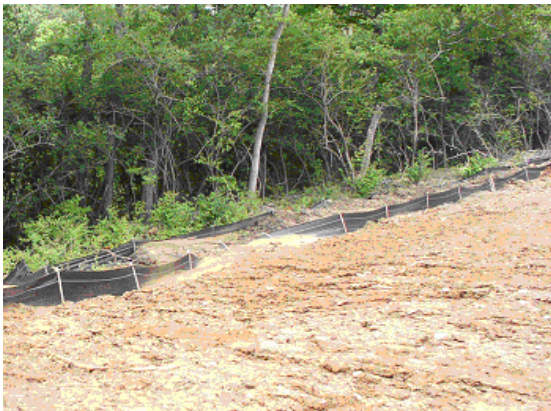
Figure 5. Silt fence inappropriately placed across contour and in area of conc. flow
