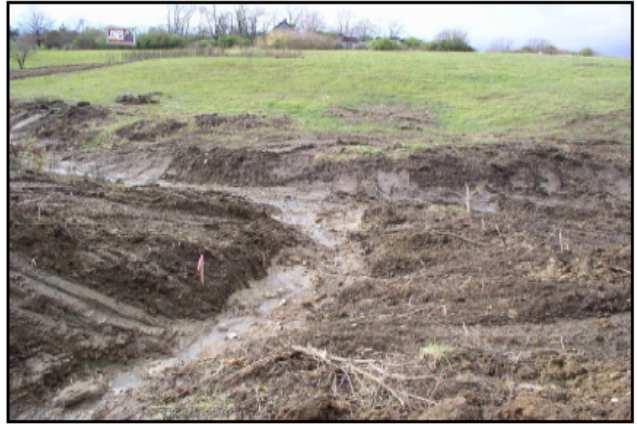
Figure 2. Confluence of drainage swale and ephemeral stream. Sediment basin should not be placed in streams. An appropriate location is just above this confluence.
