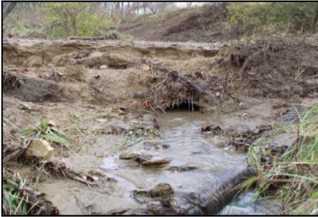
Figure 1. Pipe under temporary stream crossing has been filled with sediments from construction site. This sediment laden water discharges off-site (Looking North)
