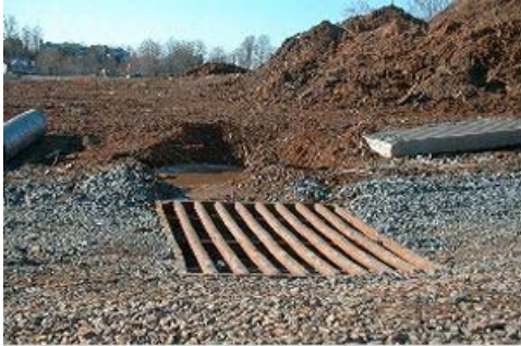
Stabilized construction entrances allow dirt to be removed from tire treads and collected as trucks leave construction sites
