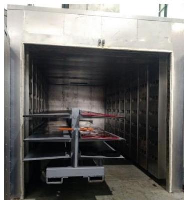
Figure A.1.10 Overnight Curing Ovens
