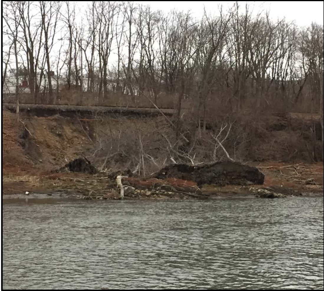
Figure 70. Photograph of rotational slump just downstream of transect D-6 (843 m ULFD) taken on November 30, 2014. The slump was first observed in the former dam pool on May 23, 2014 and occurred during a heavy precipitation event and the 6th largest flood on the Cuyahoga River on May 13, 2014.
