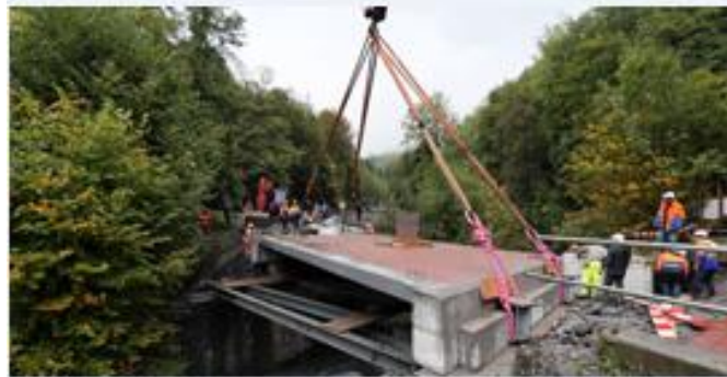
Figure 1.4 First fiber composite sandwich bridge in Switzerland. Courtesy of 3A Composites, Inc.
