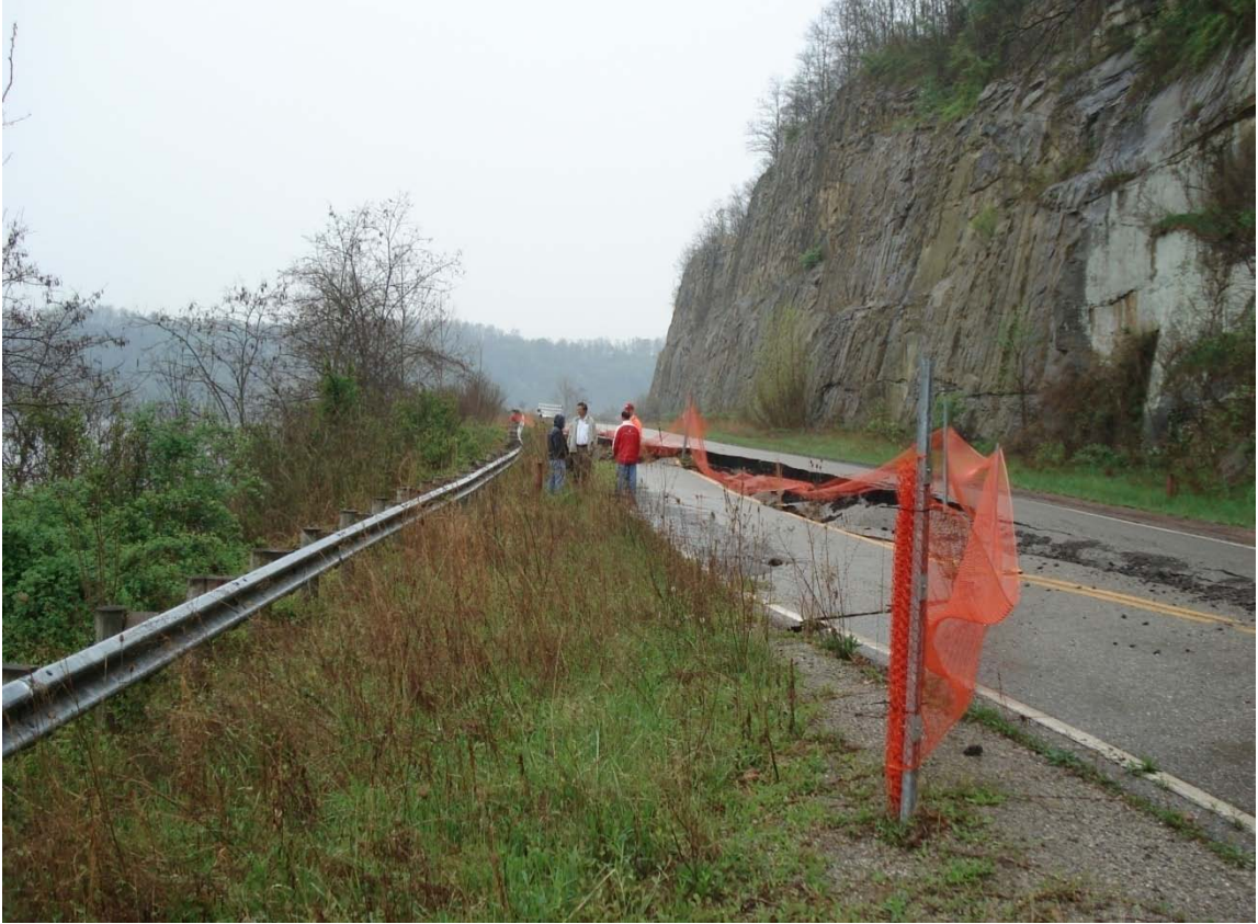
Figure 4.8: A Picture Showing the ATH Site Condition Prior to Construction of Test Drilled Shafts
