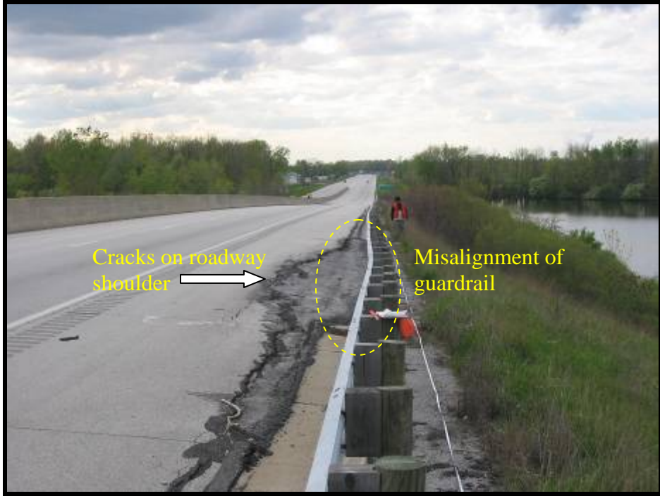
Figure 4.7 Cracks on roadway shoulder and displacements of guardrails
