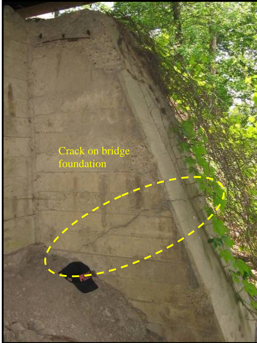
Figure 4.4 Cracks at the bridge foundation
