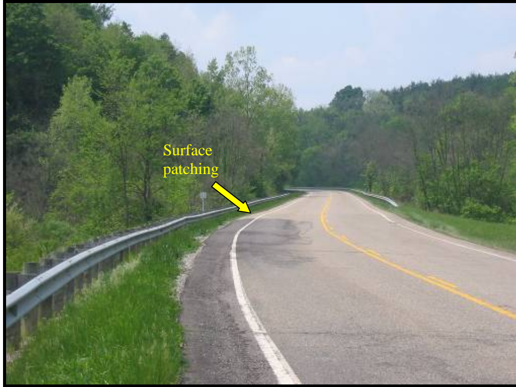
Figure 4.12 Surface patching and transverse cracks
