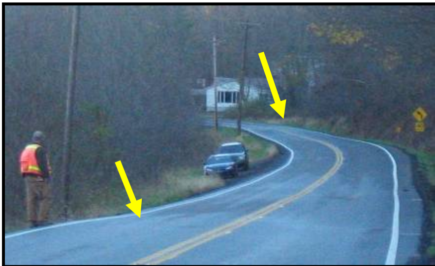
Figure 3.13 Newly paved roadway surface with evidence of failure that may not be obvious to the investigator
