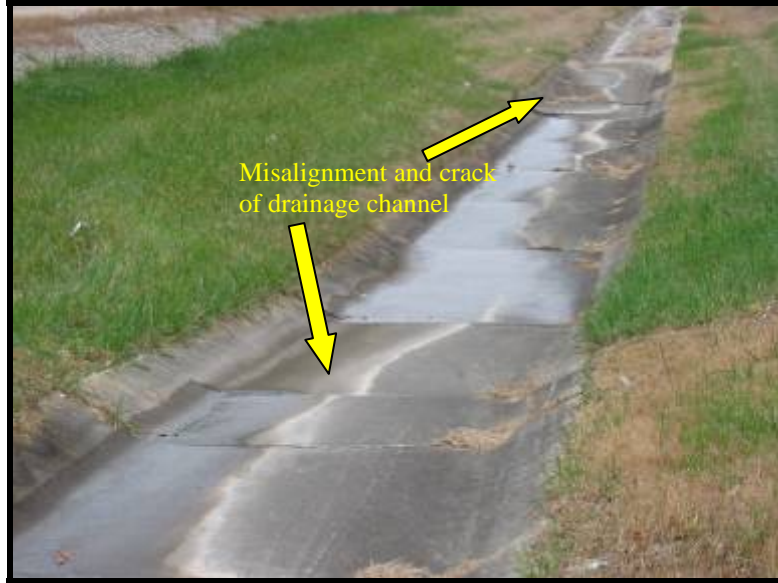
Figure 2.3 Misalignment of drainage channel
