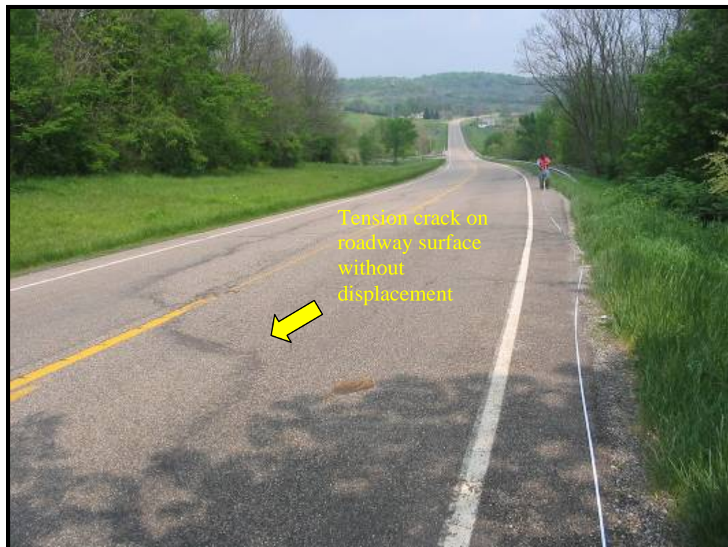
Figure 4.11 Crack line on pavement
