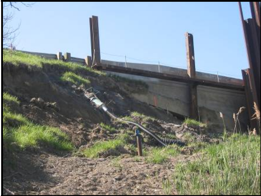
Figure 3.12 Effect of a slope failure to the stability of a bridge structure that requiring immediate response
