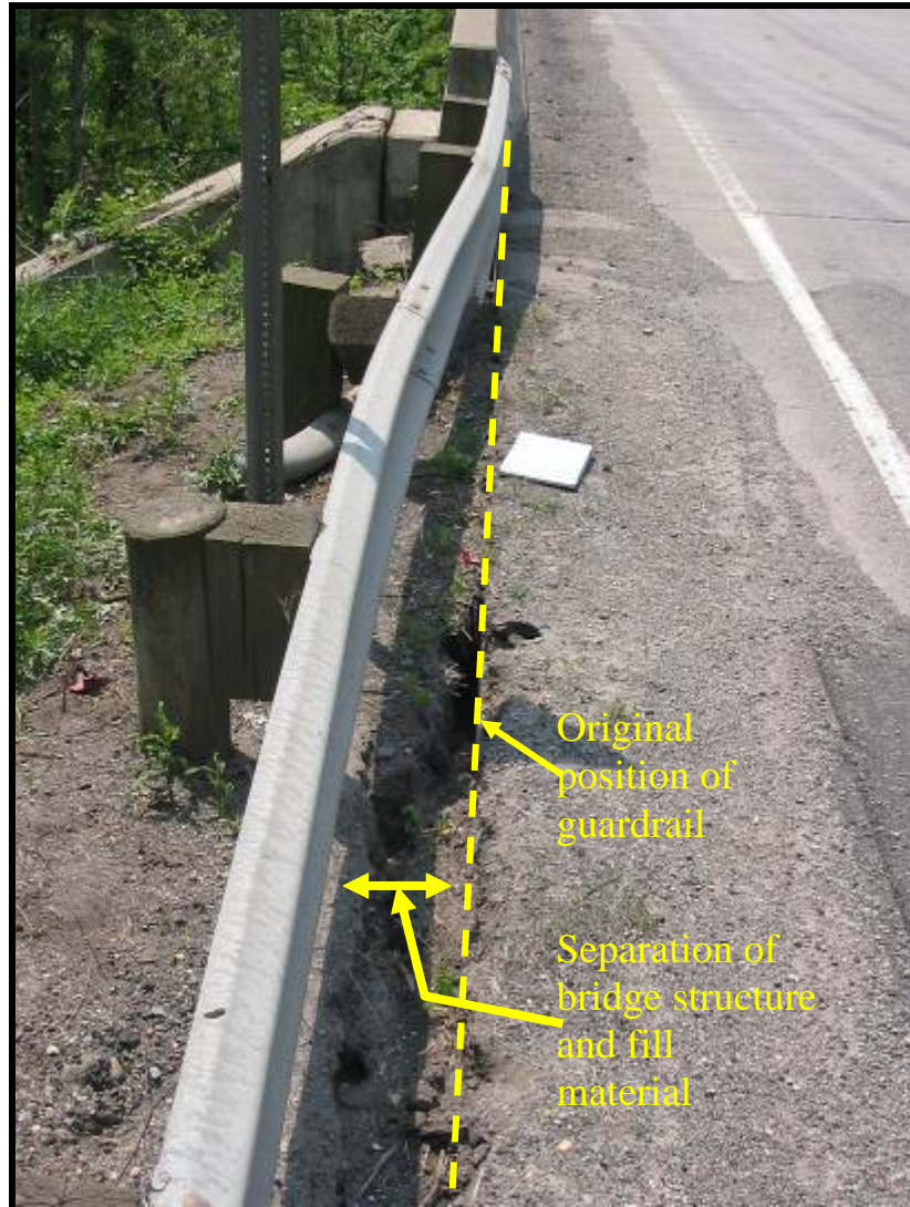
Figure 4.3 Separation between embankment and bridge structure
