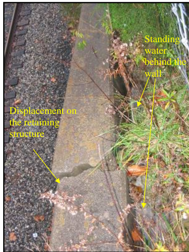
Figure 2.14 Displacement of retaining wall and standing water behind the wall
