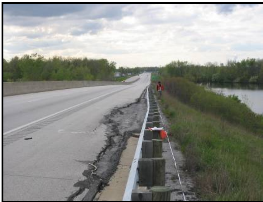
Figure 3.4 Impact on roadway shoulder with potential to affect roadway
