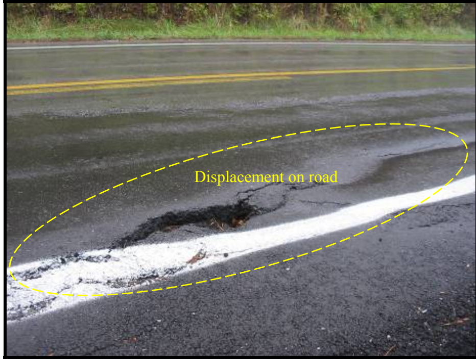
Figure 3.7 Displacement or cracks more than 3", receiving a risk score of 81
