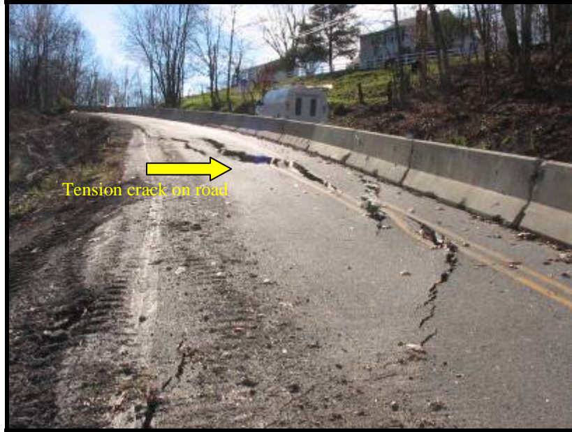
Figure 2.5 Tension cracks on road
